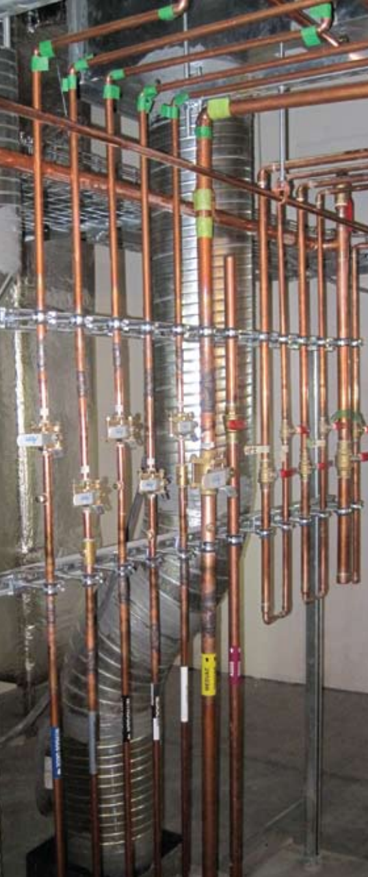
A "pipe rack" station in the interstitial area between patient floors showing the soldered domestic water lines and the taped, ready-to-be-brazed medical gas lines.
