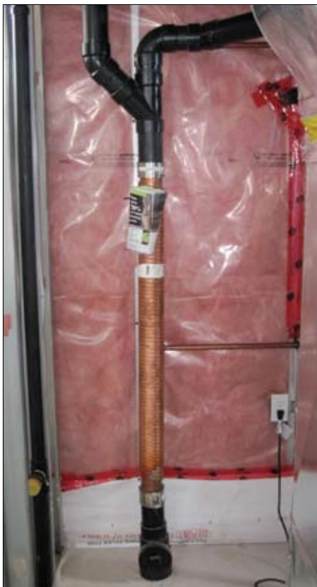
The copper Drain Water Heat Recovery Unit on the main drainage stack captures heat from warm or hot waste water which is used to pre-heat incoming water.
