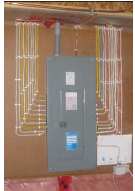
Copper power and communications wiring for the automated, energy efficient home. The pride in Gilles Michaud's quality homes is clearly evident.
