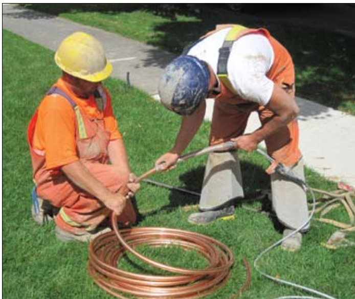
The cable and torpedo splitter are attached to the Type K copper water tube.
