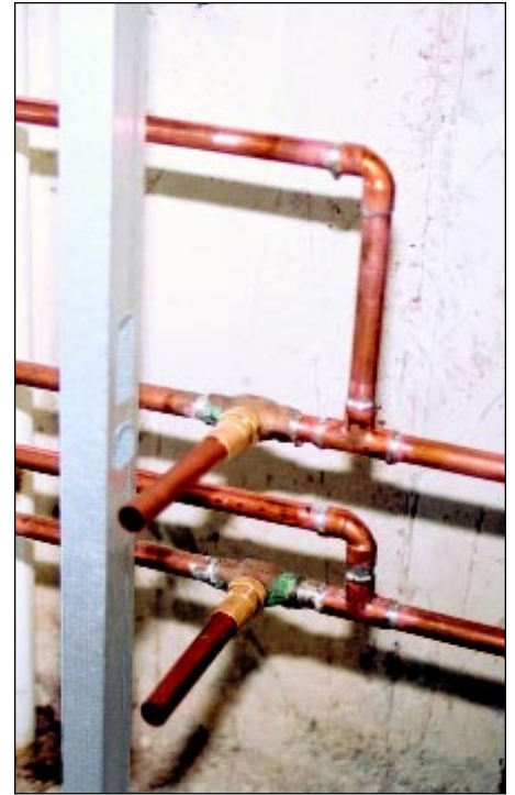
Close up of hot and cold water supply lines before application of insulation.
