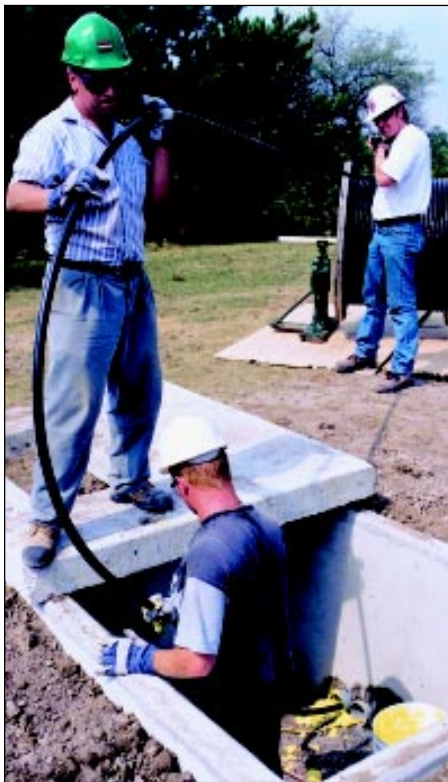
One of three 15 kV #1/0 AWG copper cables being installed in an underground conduit to bring power from the wind turbine to the grid.
