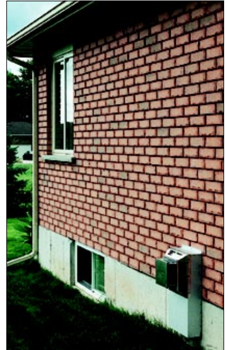
Exterior part of the direct vent for a gas fireplace in the family room of a Thornbury residence.
