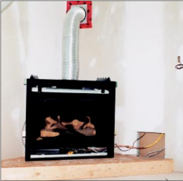
A corner gas fireplace with the copper supply line before installation of the mantel.
